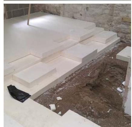
(above) The decision was taken to change the floor levels and install an insulated slab, which would also help to thermally isolate the new three storey load bearing structure from the ground and walls. 230mm of Hexatherm XPS insulation was installed to deliver a U-value of 0.094
